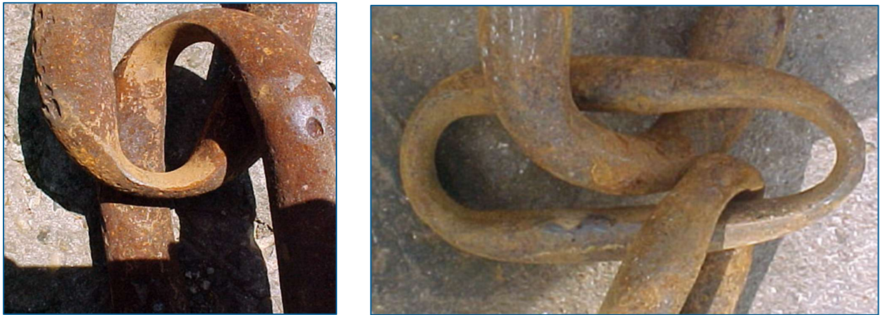
Figure 21 Abrasion and wear on mooring chains
